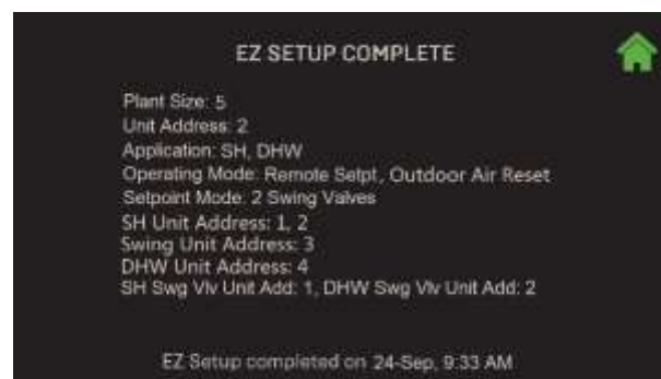
BST MANAGER, APPLICATION = SH & DHW
