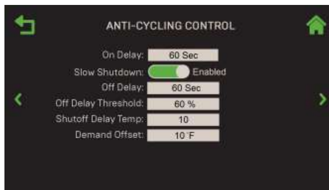
Figure 6-83 : Fire Control : Commandes Standalone Anti-Cycling
