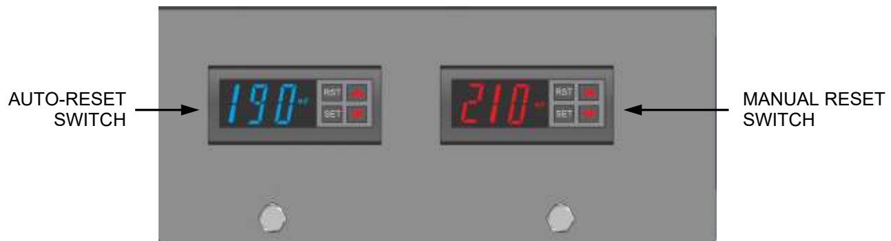
Figure 4-11: Over-Temperature Limit Switches
